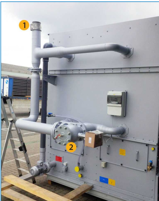
Unit with closed external piping
